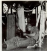
ADC Sabe Watkins, B-57 crew chief, installs rubber molding on landing gear door during phase inspection.
