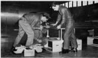
Tsgt Manuel Guerrero (left) performs sheet metal work as Ssgt Archer (center) and Ssgt Stranbury (right) assist.
